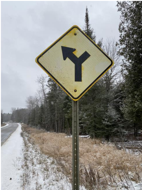
(7) Sign with almost no reflectivity left on it on Hwy 620.
